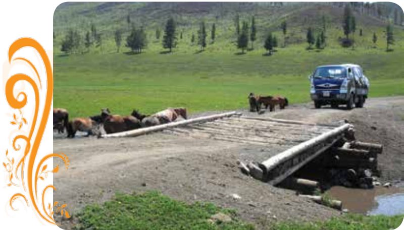
Photo 8. Khamardavaa bridge, which was repaired by the members of the “Baatar Vangiin Khishig Kholboo” NGO
